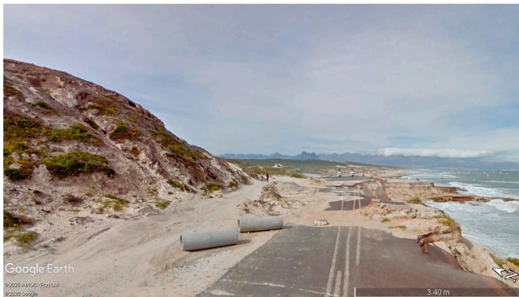
Fig. 4. Damaged part of the road due to coastal erosion Source: Authors, based on Google Earth Pro Imagery.
